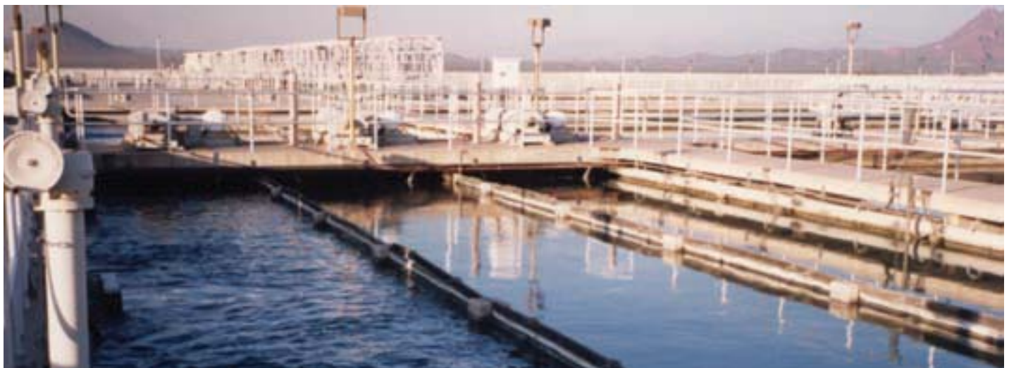
A water filtration plant where flocculators are found
